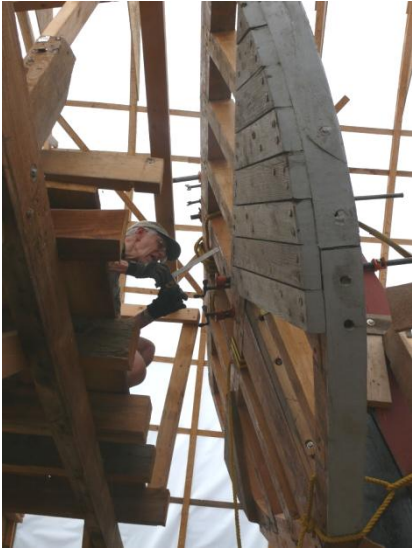
Gil Ross measures and marks the transom in preparation for drilling the through bolt holes.
